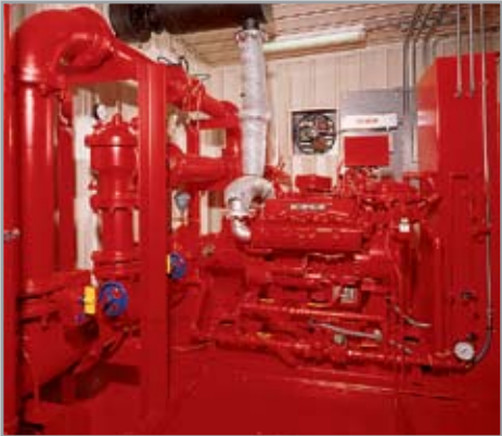
Housed Pre-Pac unit.
